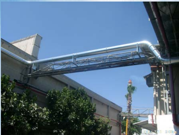
3. The pipe is crossing a road by a bridge between the 2 bldgs.
