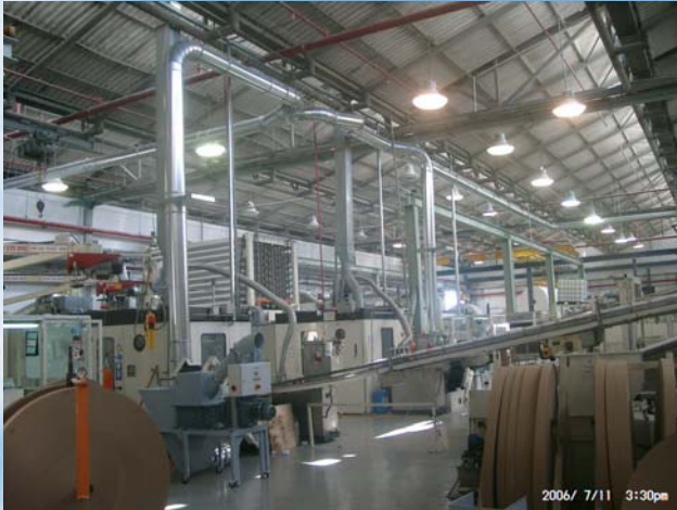
5. The pipe goes down to 2 of the production lines
