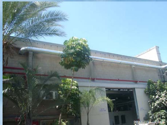
4. The pipe is between the end of the bridge till the entrance hole to production bldg.
