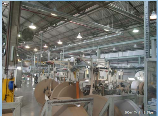
6. The pipe towards the third production line
