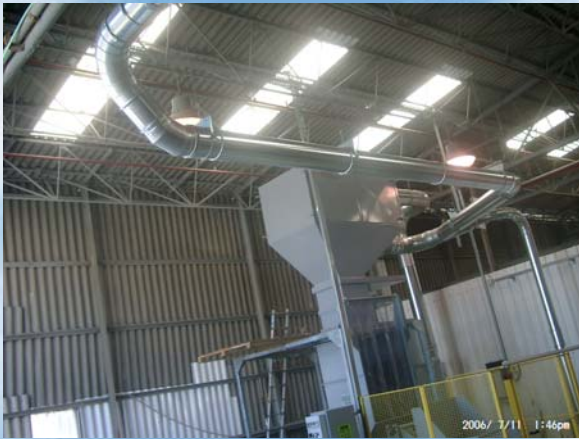
1. Outlet of the pipes from the separator towards the 3 production lines, which located in another bldg.
