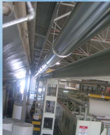
2. Long straight pipe towards the second bldg. where the 3 production lines are located
