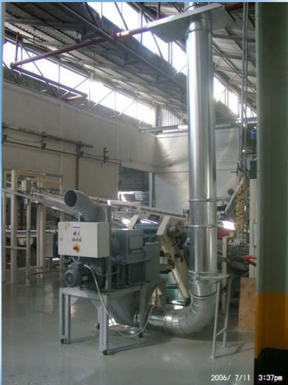
7. Connection of the pipe to a suction station. The other 2 are the same
